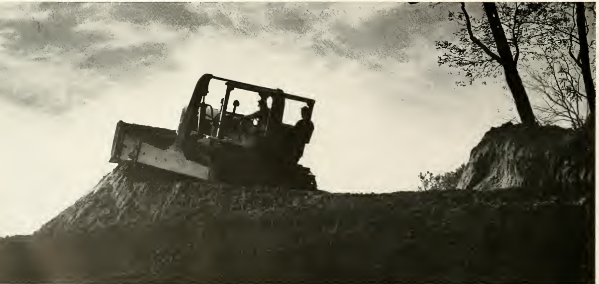
This picture of a bulldozer in action symbolizes the building program which continued all summer.
